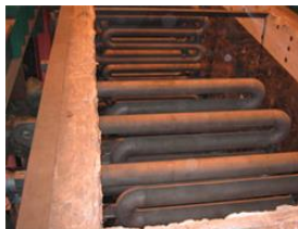
Radiant tubes in an indirectly heated continuous furnace
