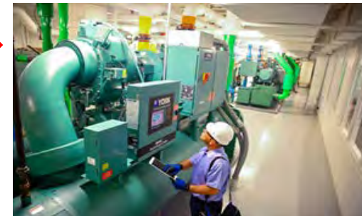
Equipment with embedded controls
