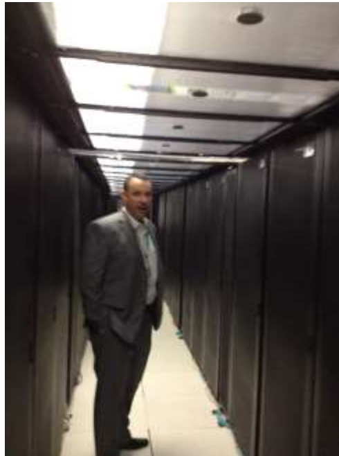
APC Hot Aisle Containment (with in-row cooling)
