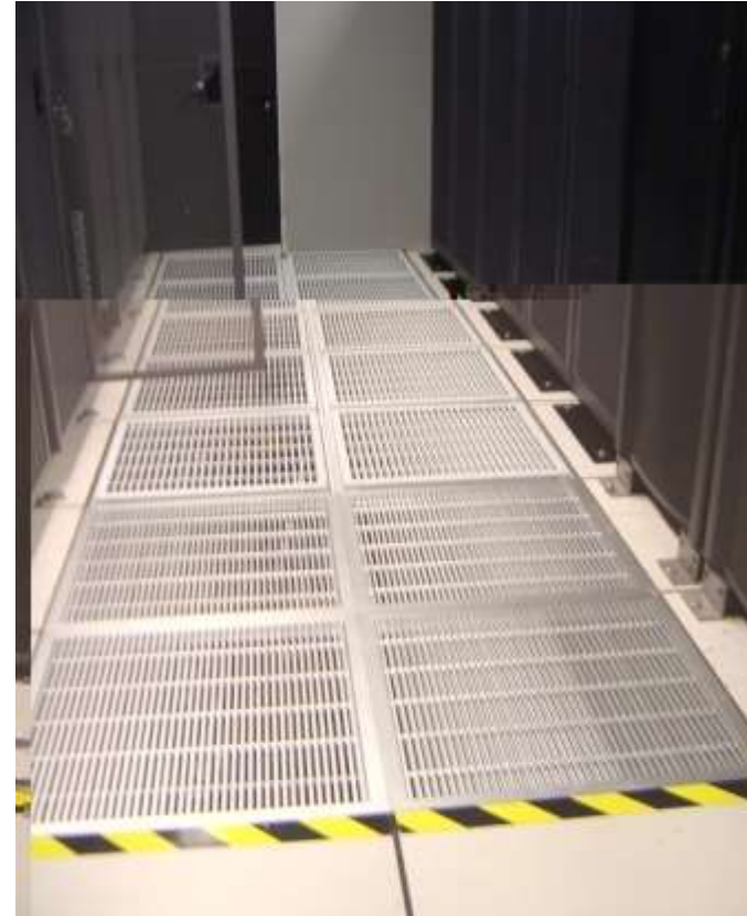
High-flow tiles reduced air pressure
