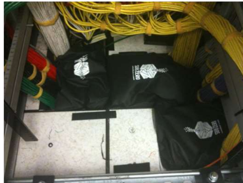
Sealed cable penetration
