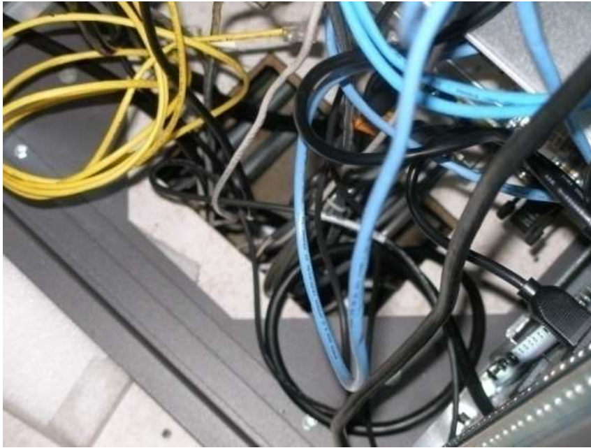
Unsealed cable penetration (inside rack)
