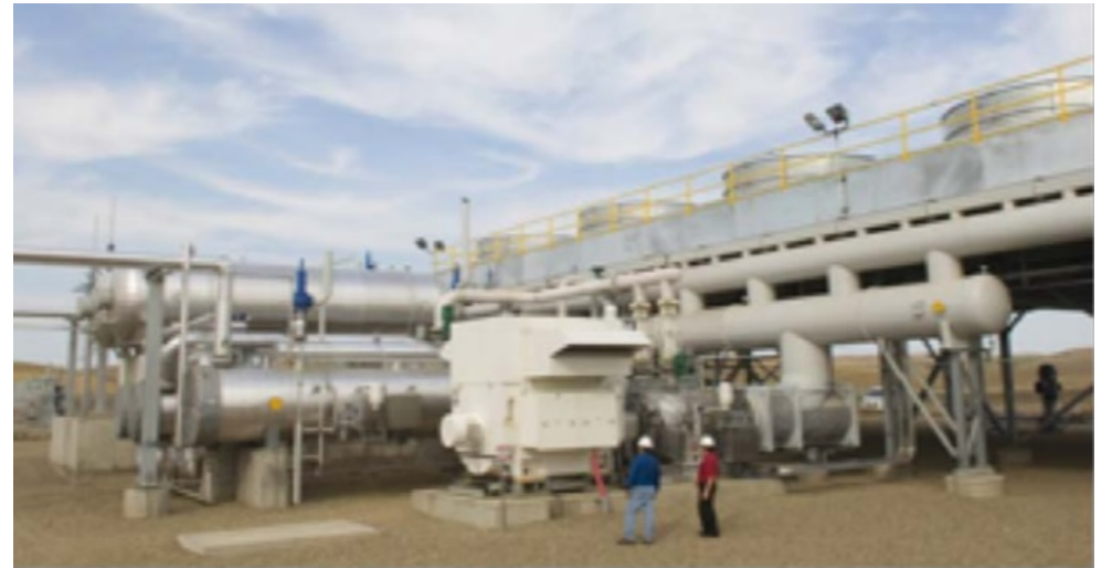
Northern Boarder Pipeline, North Dakota
