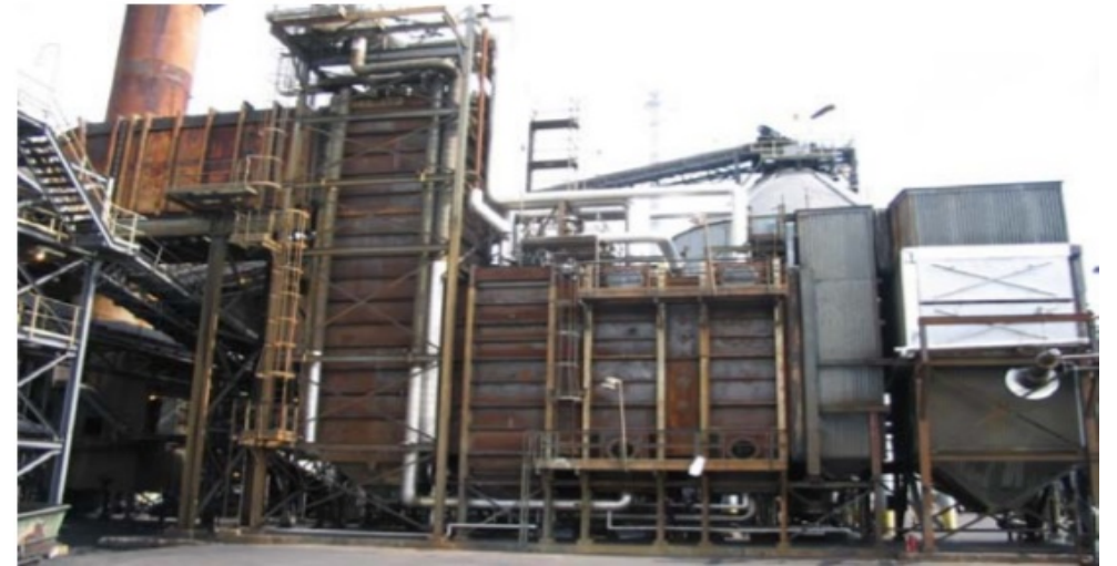
Port Arthur Steam Energy/Oxbow Corp, Texas
