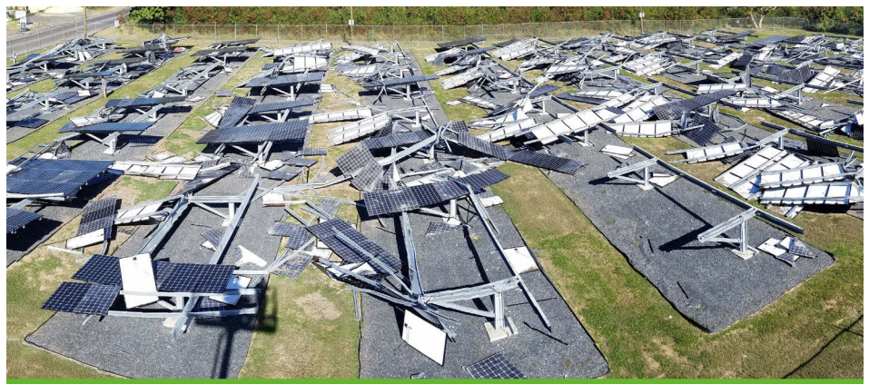
Figure 1. Unsuitable clamping fasteners lead to total photovoltaic system loss during a 2017 hurricane. Photo by Gerald T. Robinson, LBNL.
