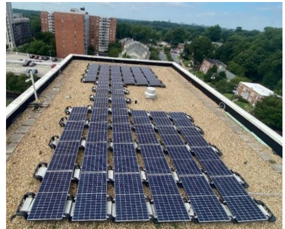
Solar PV installation at Blair Office Building
