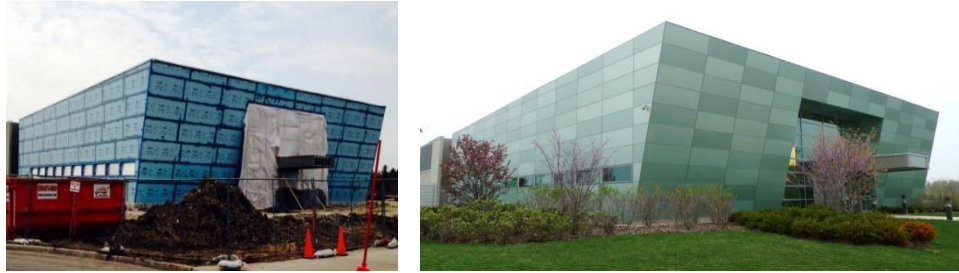
Figure 5. Front of the Homeland Security Training Center. The picture on the left shows exterior insulation that was sealed at its joints with LIQUIDARMOR™ CM Flashing and Sealant. The picture on the right shows the finished building clad with metal curtainwall panels.
