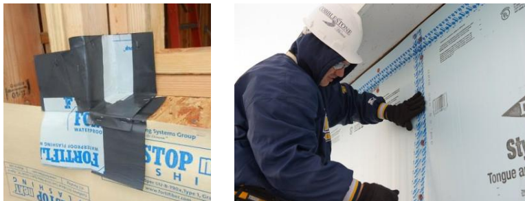
Figure 1. Tape used to flash window rough openings (left) and to seal joints between boards (right).
