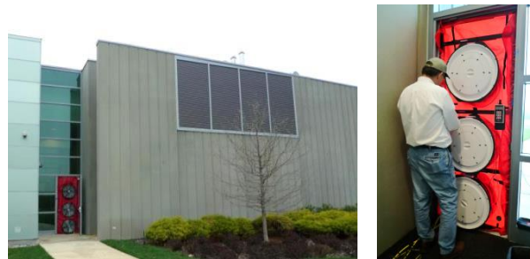
Figure 8. Blower door setup on west side of building. Left picture shows the louvers that provide fresh air and that were closed with mechanical dampers during the blower door test.
