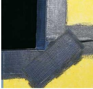
Figure 2. Coating and reinforcing mesh flash the rough opening of a window and seal gaps between exterior grade drywall wall sheathing.
