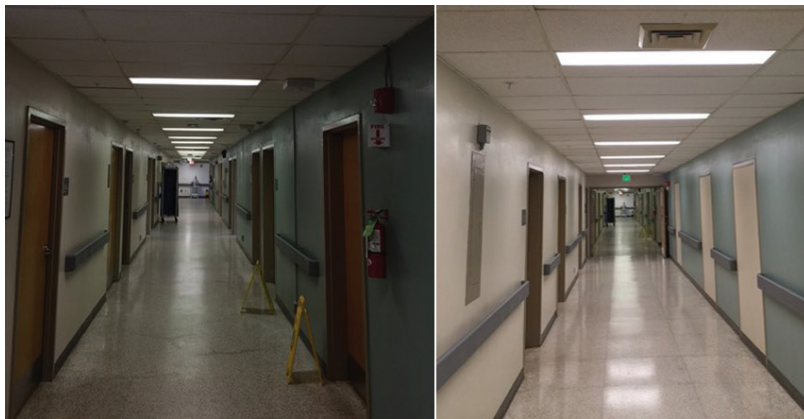
CHRISTUS Health replaced the fluorescent lamps with LED lamps in 16,400 troffers across 10 hospital sites, totaling 5.5 million square feet of facility area, for annual energy savings of 4.71 million kWh and cost savings of $300,000. Photo courtesy of CHRISTUS Health.
