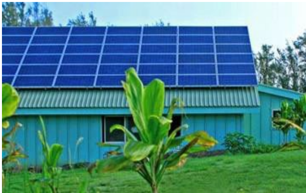
26 kW rooftop PV system that supports the retreat's electricity needs
