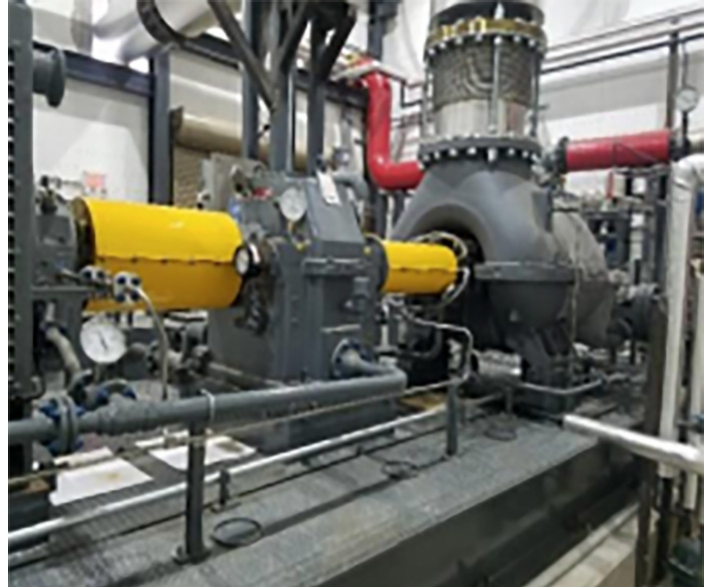
Backpressure Steam Turbine Installation at an Ethanol Plant in Lena, Illinois.
