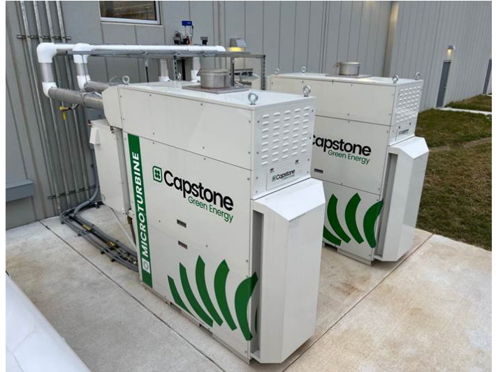
Microturbine CHP Installation at a Commercial Facility. Photo courtesy of Capstone Green Energy
