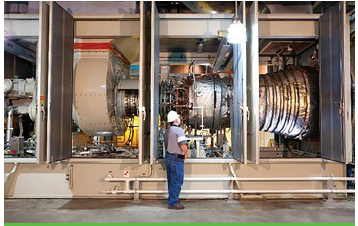
Gas Turbine Installation at a University. Photo courtesy of Solar Turbines
