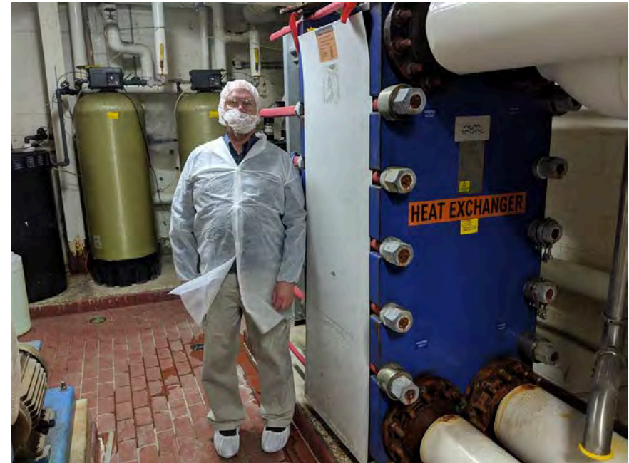
New Heat Exchangers
