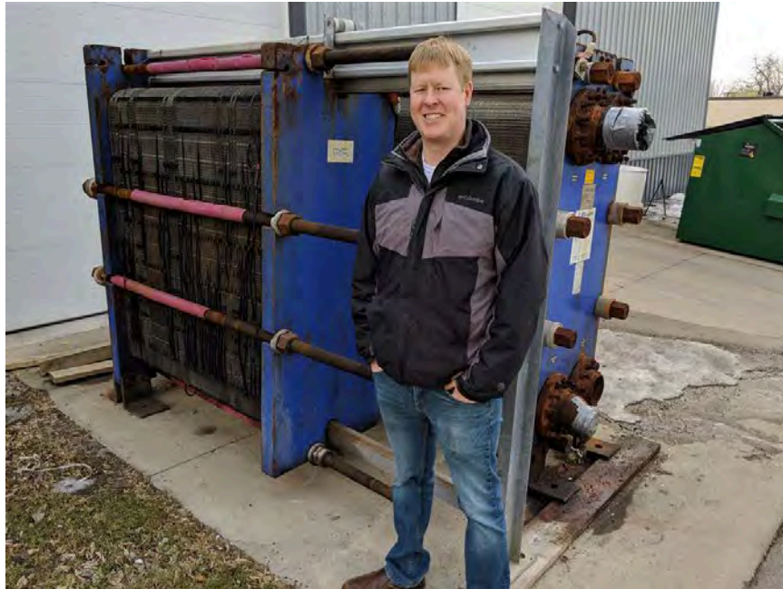
Old Heat Exchangers
