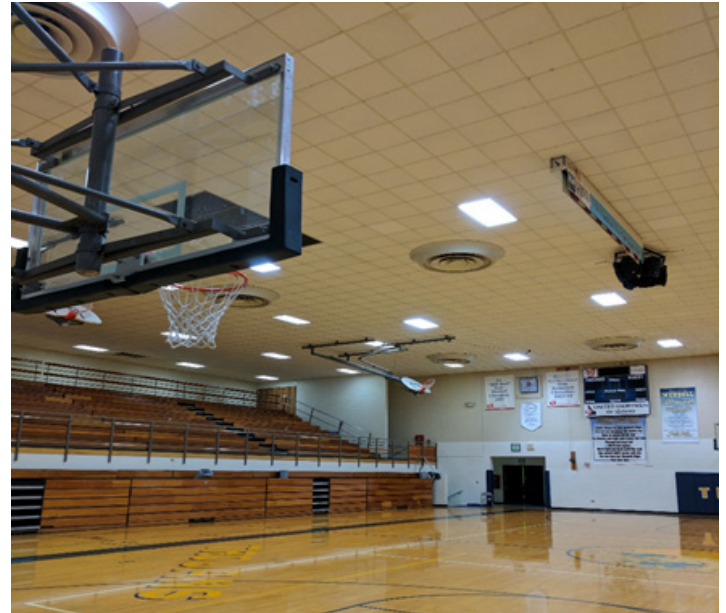
HVAC timers in all buildings, especially the gymnasium, save energy for the district. Photo credit: Wendell School District.
