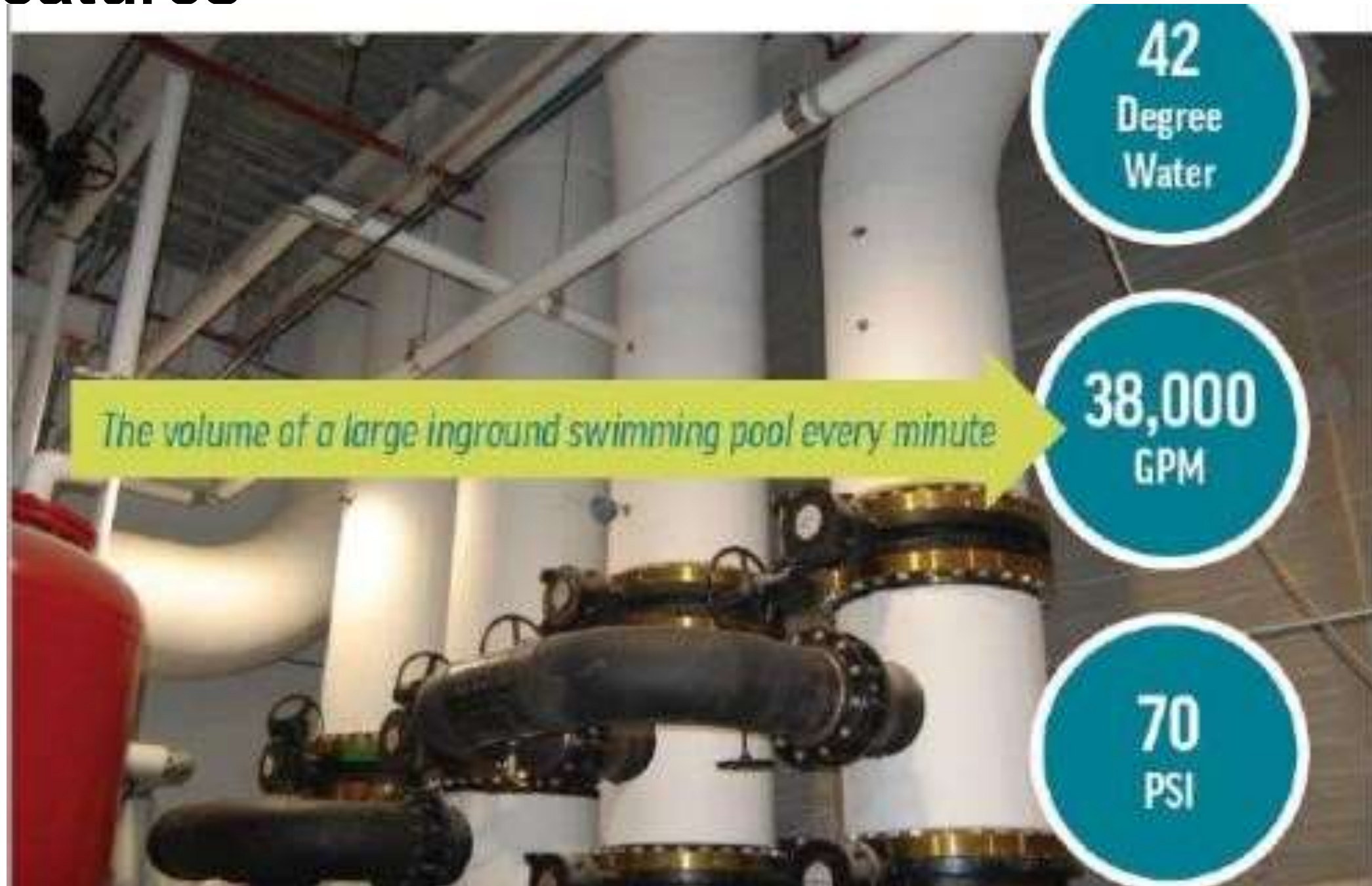
Chilled water distribution through 42" supply and return lines
