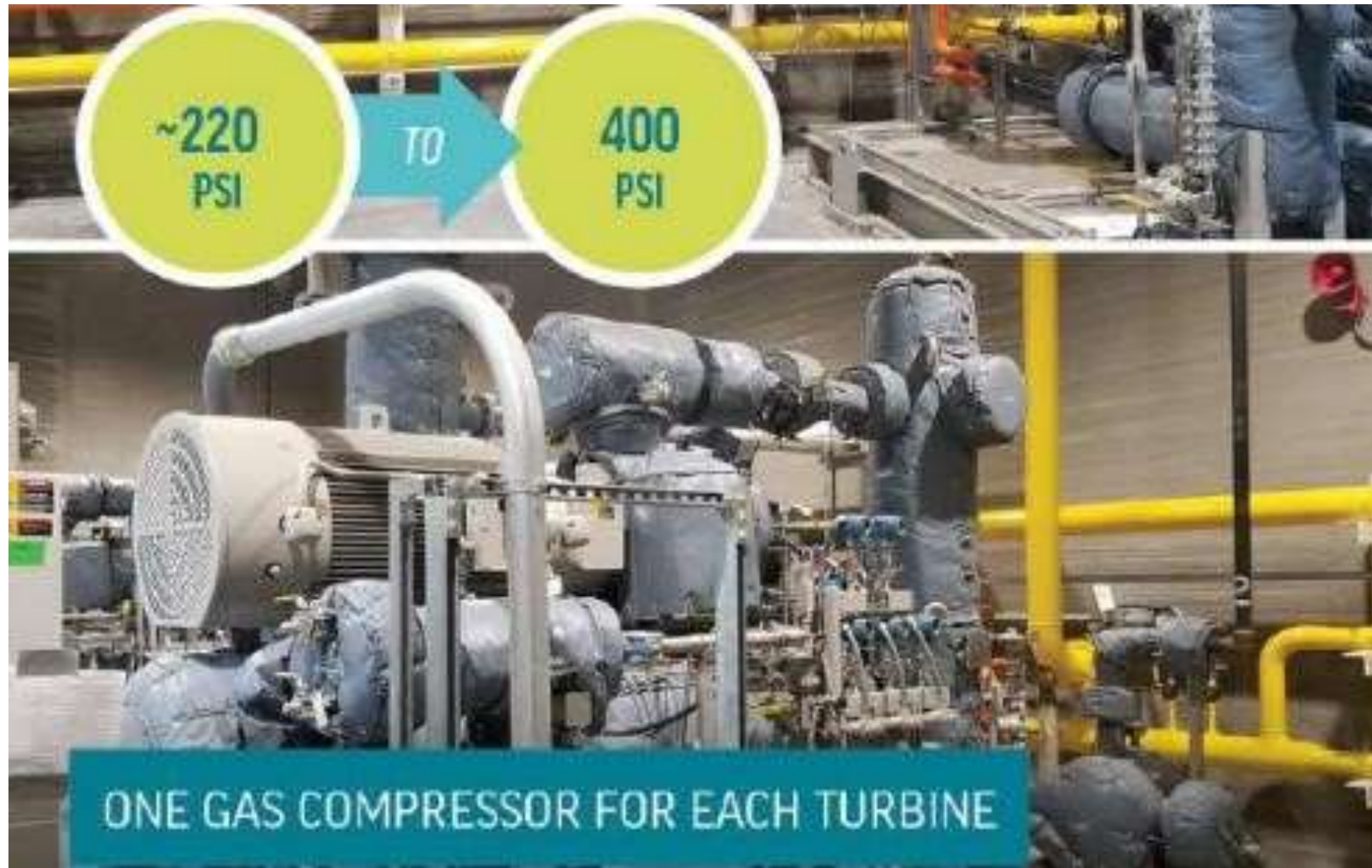
Vilter Gas Compressors
