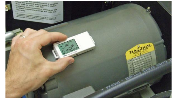
Run time loggers to monitor pump operations
