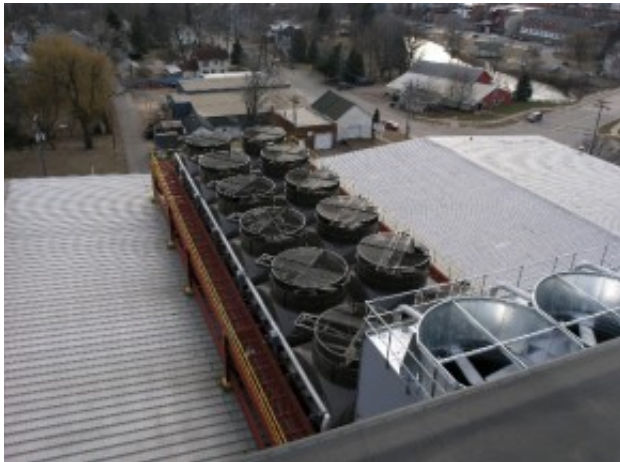
Hot oil heat exchangers
