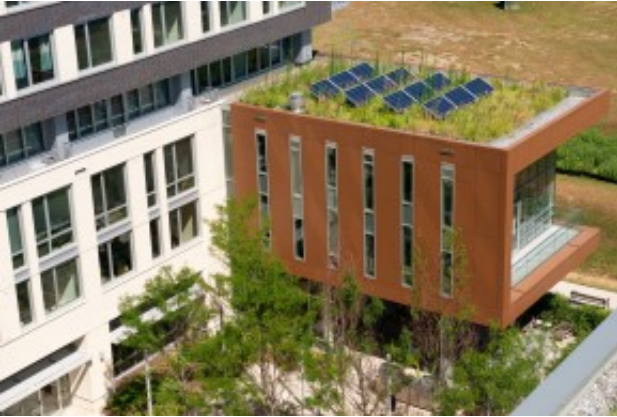
Solar racking system
