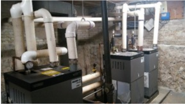
Washington Columbia's New Boilers
