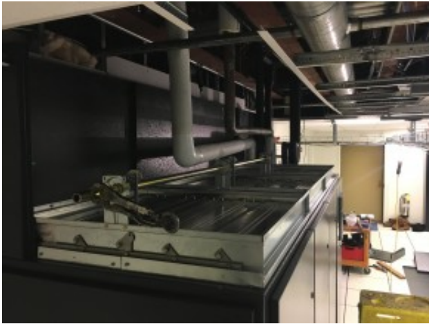
CRAC Backdraft Damper
