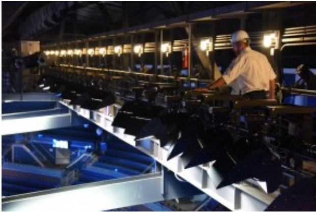
New LED sports lighting fixtures
