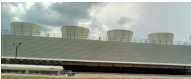
Chiller Cooling Towers
