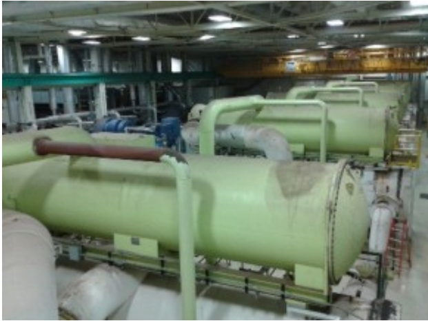
Lineup of 6,750-Ton Chillers
