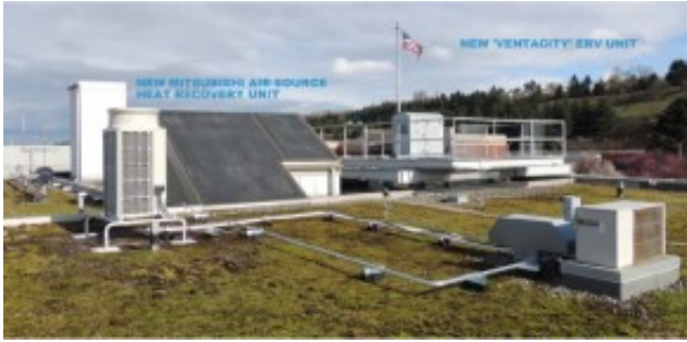
New air-source heat recovery and energy recovery ventilation (ERV) units
