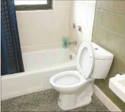
New instantaneous gas hot water heaters and water conserving bathroom fixtures are among the improvements now installed at the homes of Palatka Housing Authority residents.
