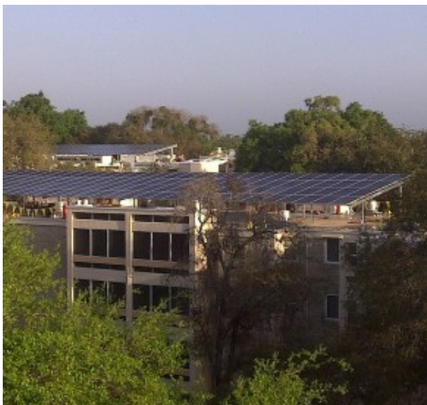
Solar Panels at J.L. Young Gardens
