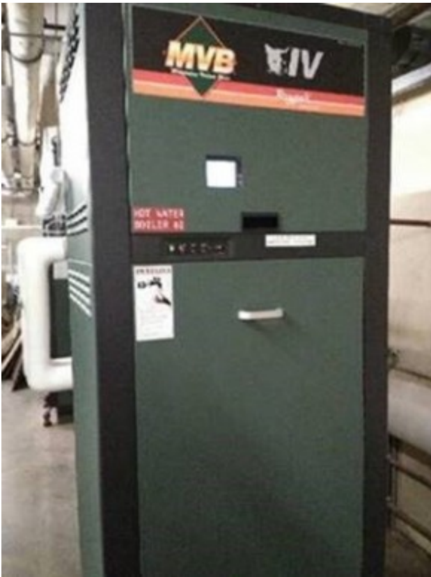
Forced Air Raypak Boilers
