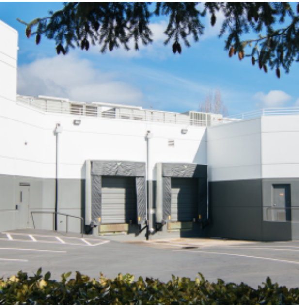
Rear of Nike Miler building, view of new HVAC Units
