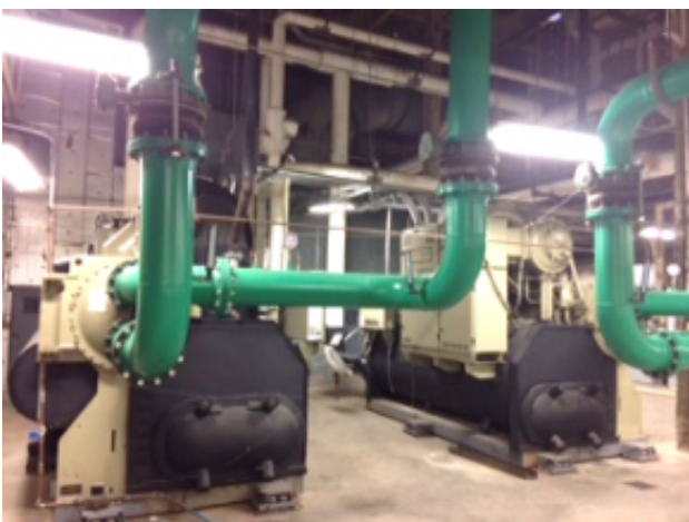
Two highly efficient Trane 500-ton chillers
