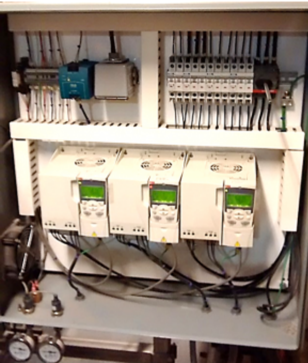
Control panel for triplex booster system
