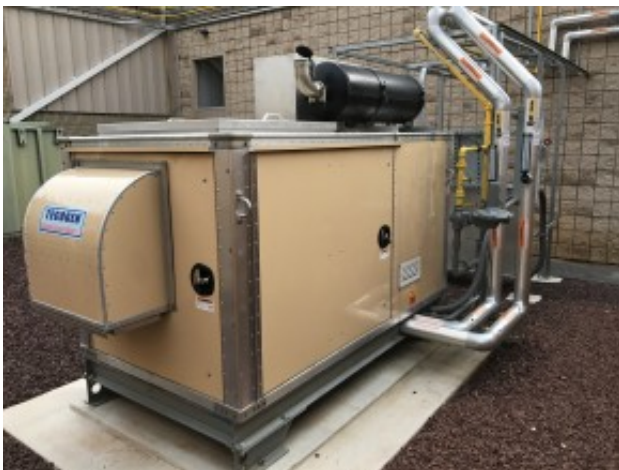
60kW combined heat and power generator.
