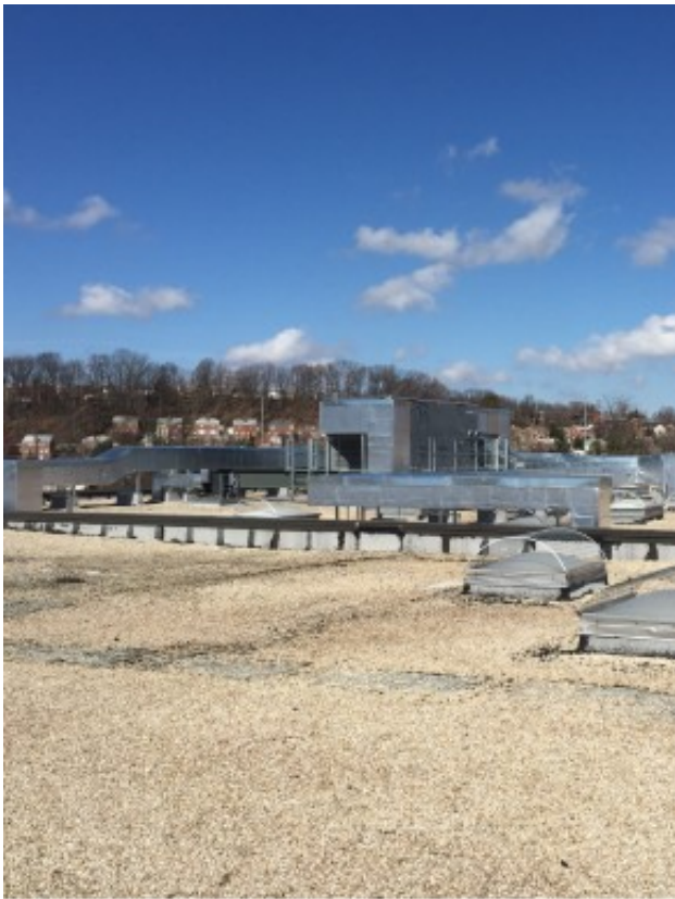
Equipment Bureau, Rooftop Units
