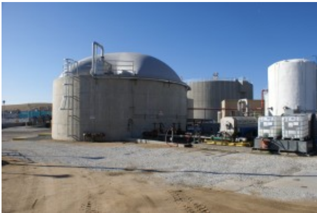
Digester tank and recuperative thickener
