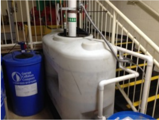
Condensate recovery returned to cooling tower
