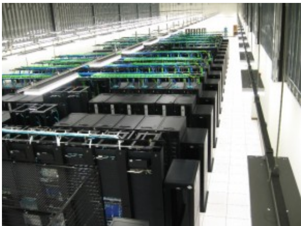
Data Hall Before Containment
