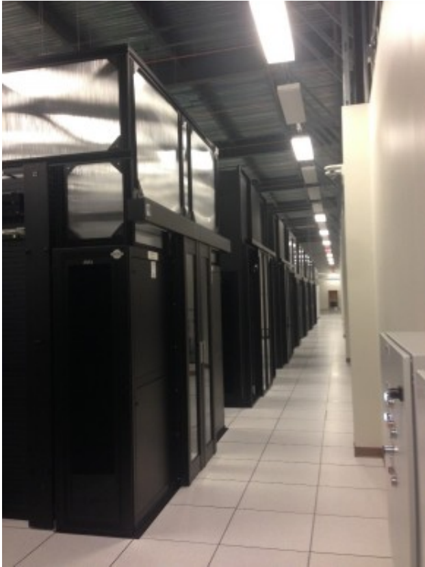
Close-up View of Containment System
