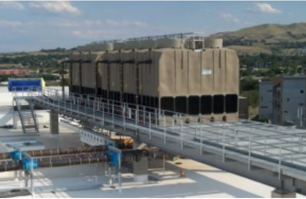
Evaporative Cooling Towers
