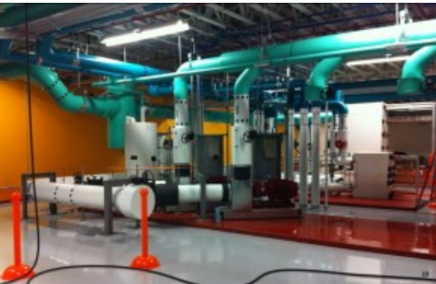
Mechanical Equipment Room
