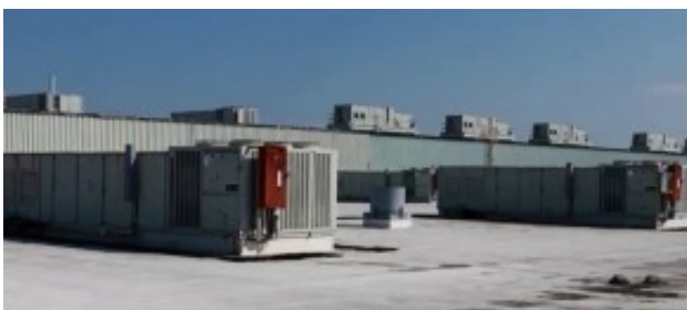
GE's upgraded HVAC units
