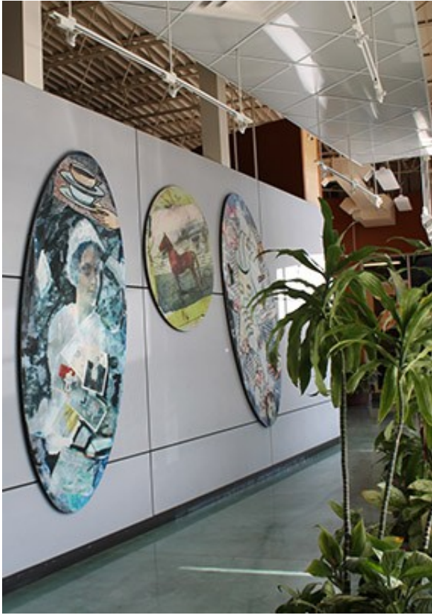
Entryway lights off due to daylighting
