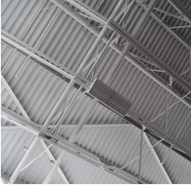
LED High Bay Fixtures Above Gym Floor
