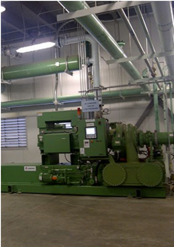
The compressor room at the Milford plant
