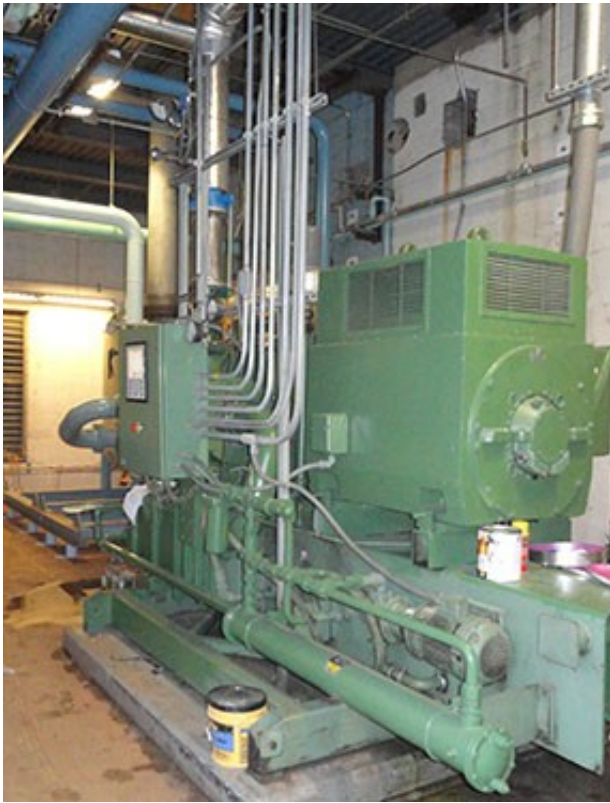
A compressor used at the Milford plant
