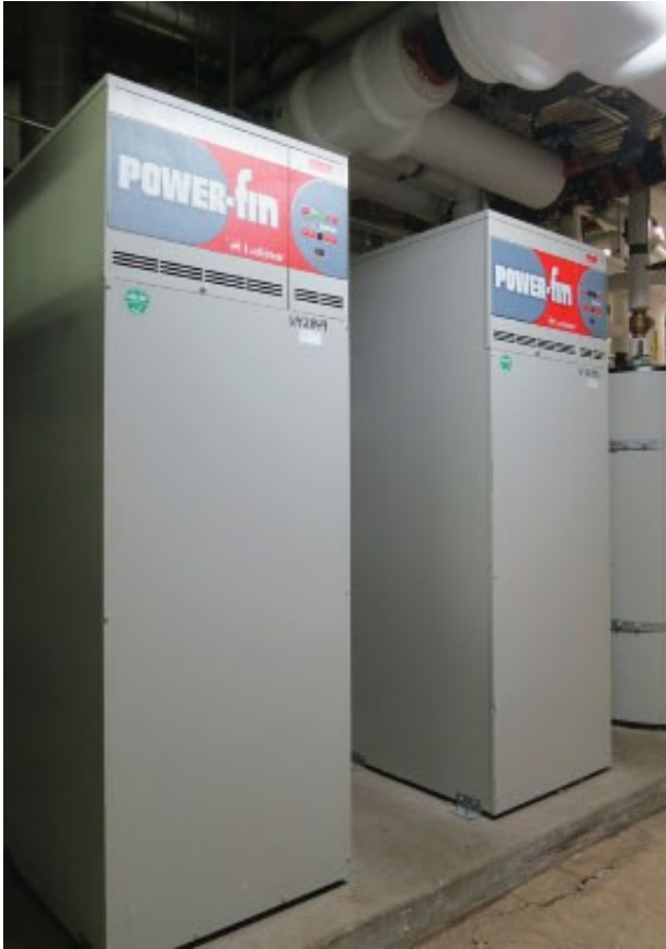
High efficiency boilers
