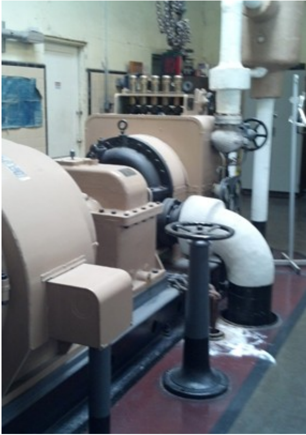
Old boiler from 1950's
