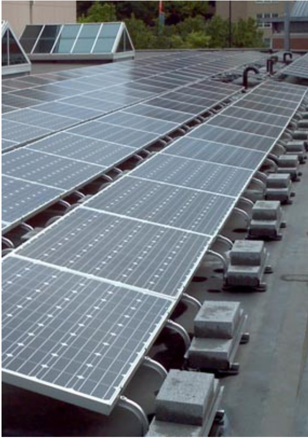
90 kW rooftop solar PV system
