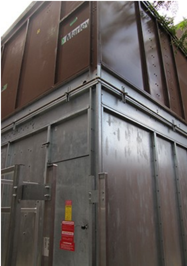
New cooling tower #1
