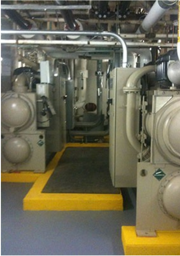
Twin, dual-compressor Turbocor chillers
