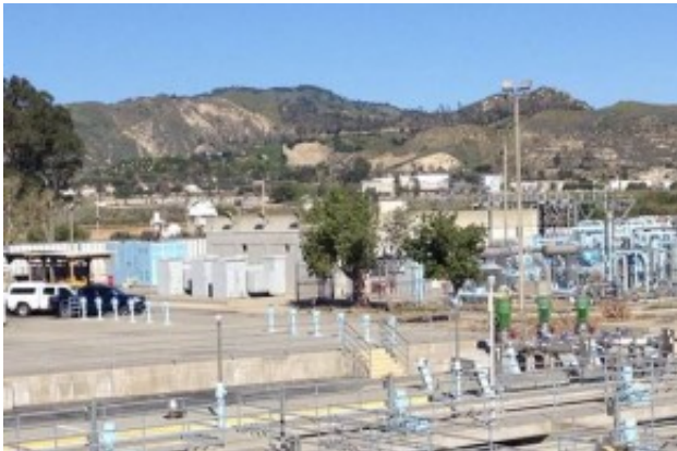
Los Angeles aqueduct filtration plant, Sylmar, California
