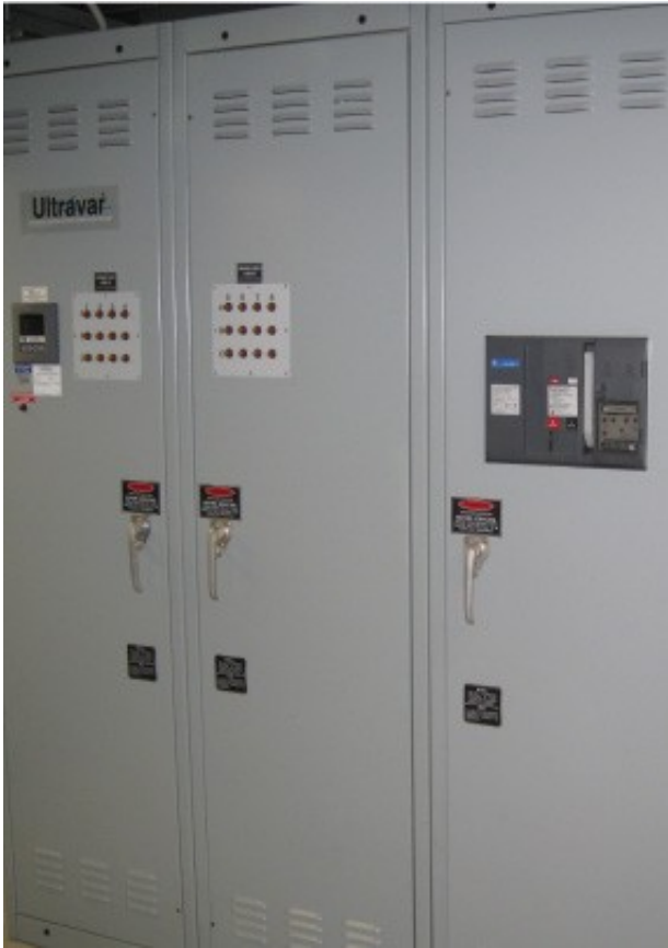
Capacitor bank improves power factor
