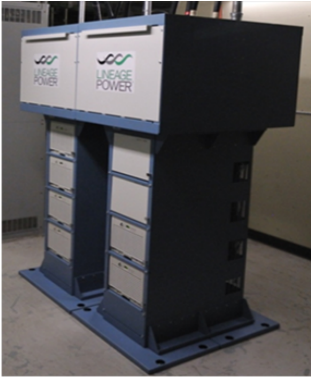
Ferro-resonant rectifiers replaced with switch mode rectifiers
