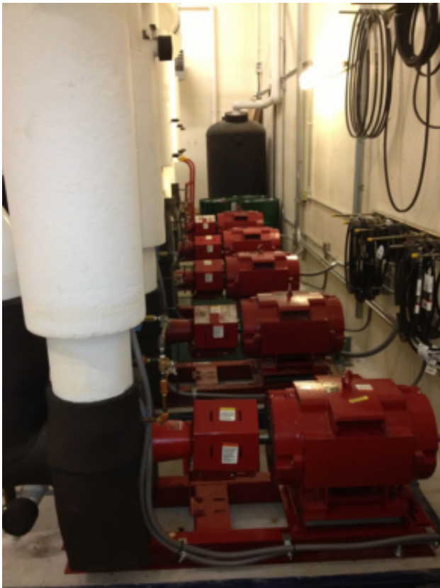
Chilled water pumps with VFDs
