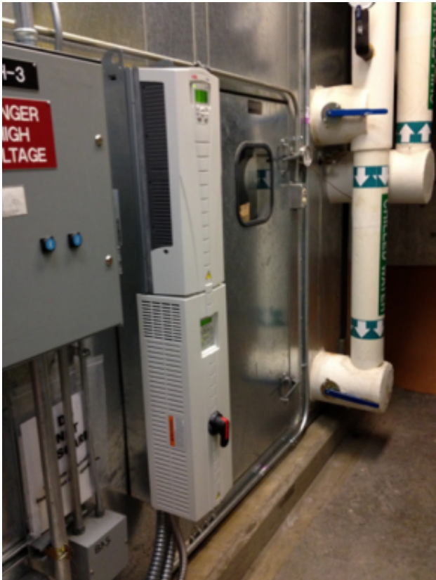
VFDs on computer room air handler units
