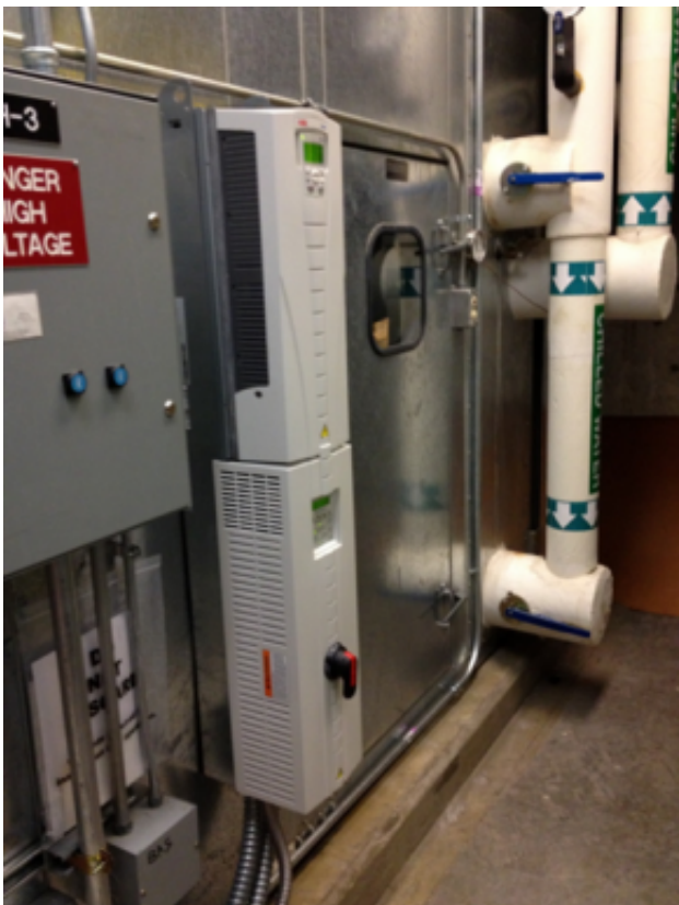
VFDs on computer room air handler units
