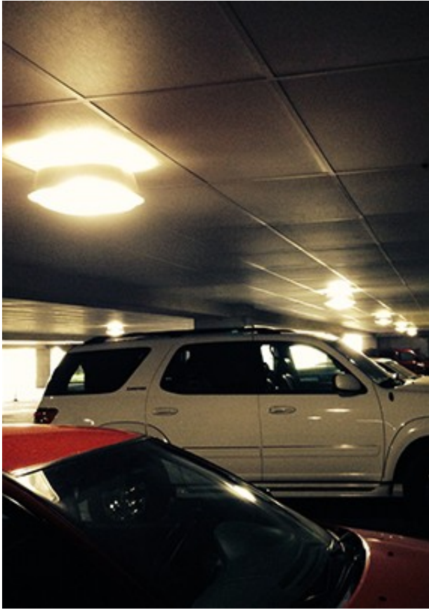
Underground parking lighting
