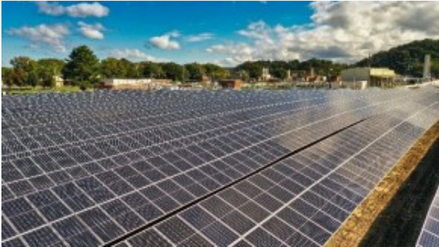
Moccasin Bend Environmental Campus Solar Panels
