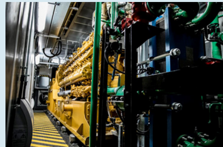
The Rimco Cat CG170-20 generator is providing 2 MW of power to the processing facility and warehouse.
